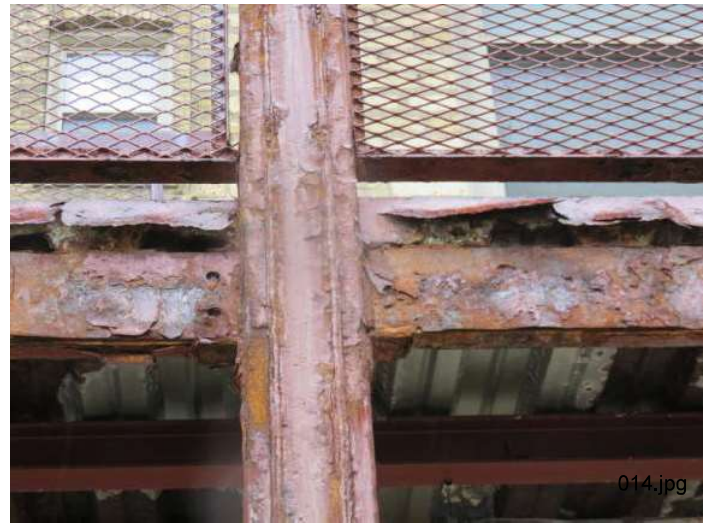
Photo: 14 Connection requires shoring
