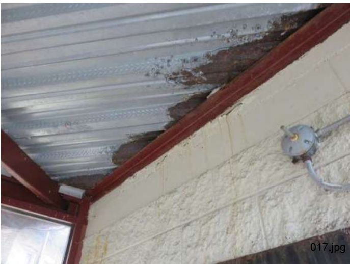
Photo: 17 Deck corrosion in elevator lobby
