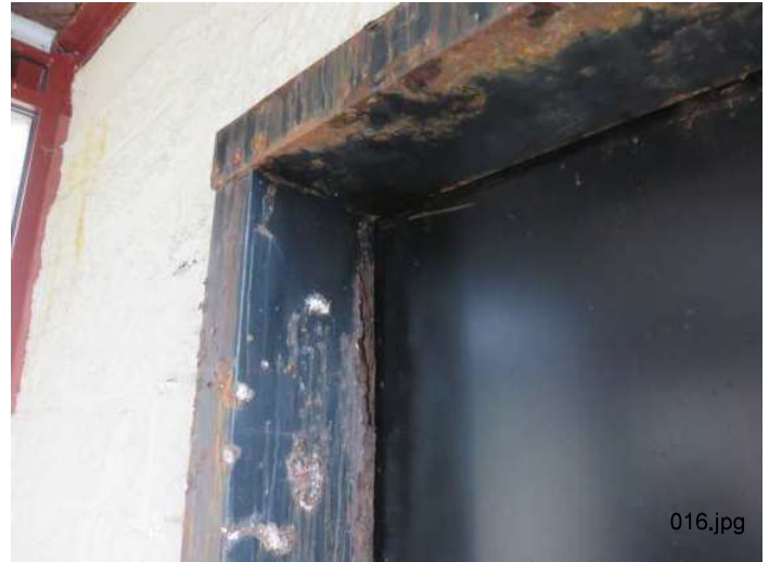
Photo: 16 Corrosion of elevator door frame
