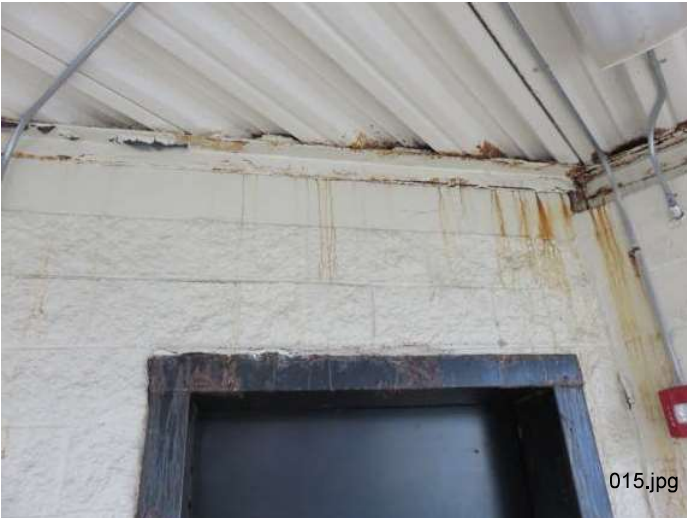
Photo: 15 Staining in elevator lobby
