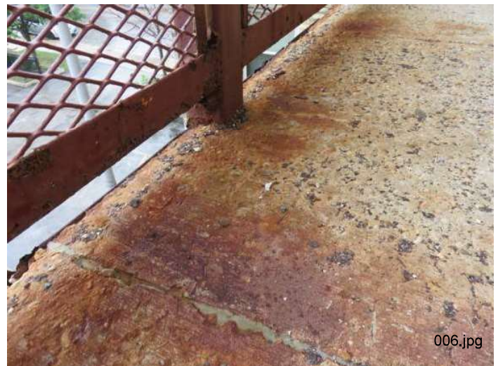
Photo: 6 Typical staining and scaling
