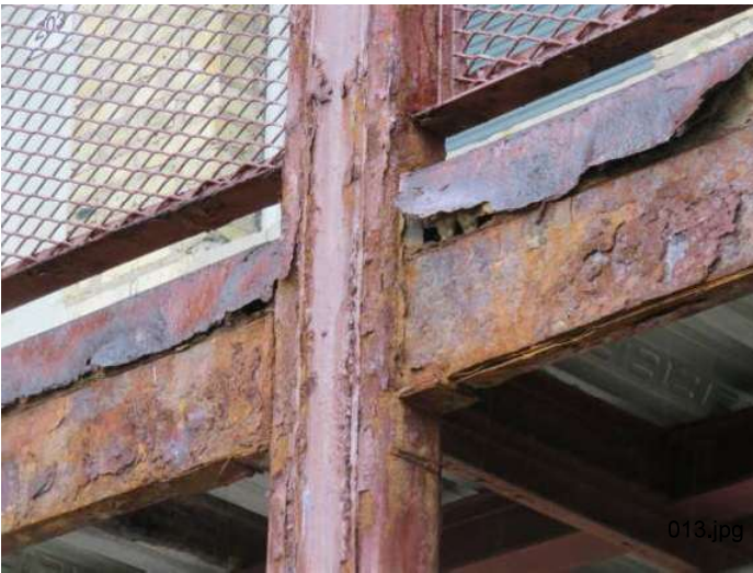
Photo: 13 Connection requires shoring
