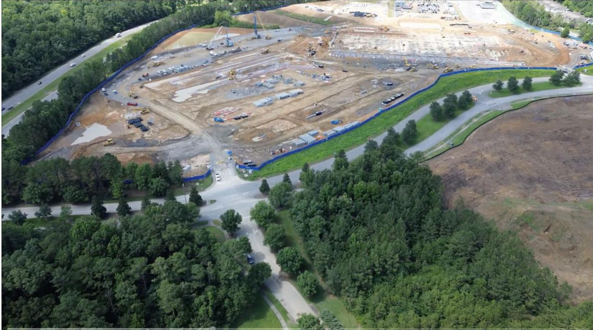
Figure 1. Aerial photograph of the BHM01 “AI Factory” construction site as of June 18, 2026, showing site clearance, mass grading, foundation and caisson work, cranes, and heavy equipment within approximately 800 to 970 feet of Plaintiffs’ homes.
