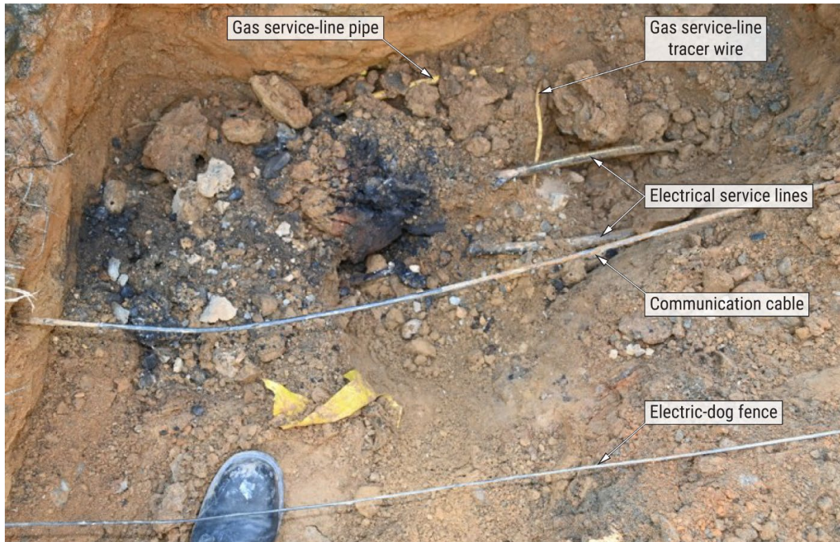
Figure 3. The accident trench.
