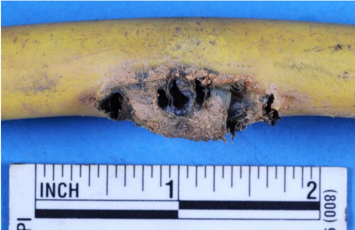
Figure 4. The “blister” on the accident service-line pipe.
